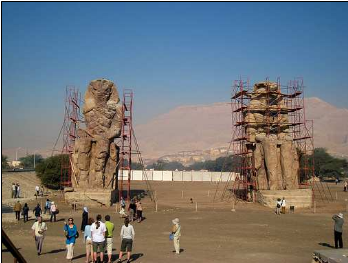
In Luxor, the Colossi of Memnon came close to toppling over, but did not. They had to be braced with scaffolding and repaired.
